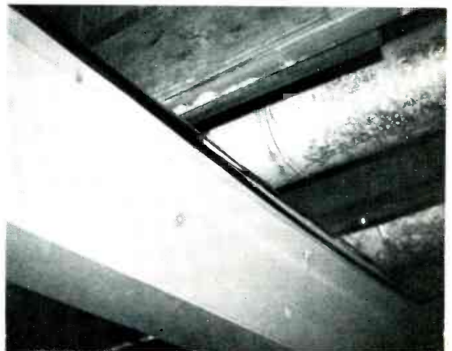
Fig. 11 Unshielded lead-in and rotator cable are routed side by side along a steel I-beam and across two warm-air heat ducts—examples of poor installation practices.
